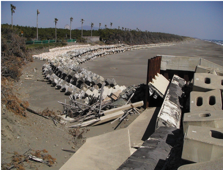
Photo 1 Erosion at the north end of coastal revetment, Sumiyoshi Beach (March 29, 2006)
